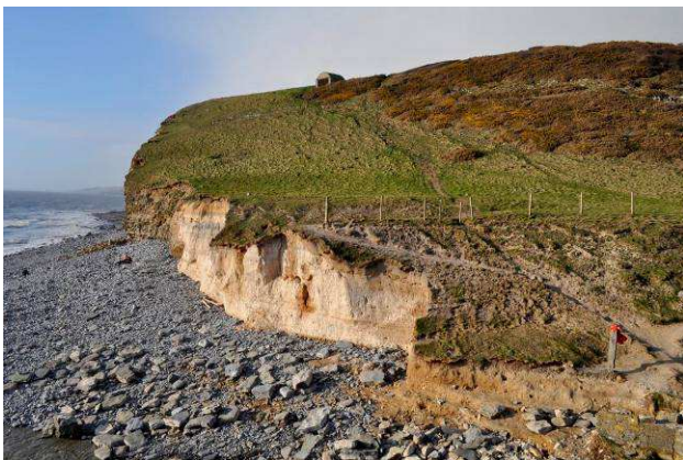
Figure 49. Cliff erosion in winter 2013/14 threatening MG5b sub-community of vegetation at Cwm Nash, South Glamorgan (Christina Byrne, Natural Resources Wales)
