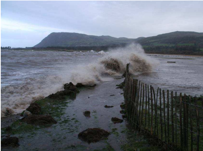
Figure 20. Overtopping of the floodbanks at Morfa Madryn, Llanfairfechan (John Ratcliffe, Natural Resources Wales. 5 th Dec 2013).
