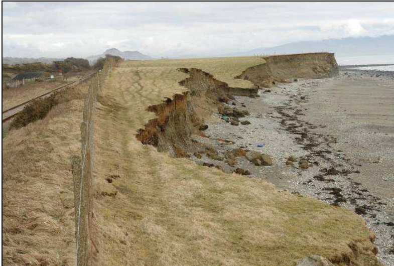
Figure 7. Erosion at Glanllynau is likely to lead to casework with Network Rail (Stewart Campbell, Natural Resources Wales).
