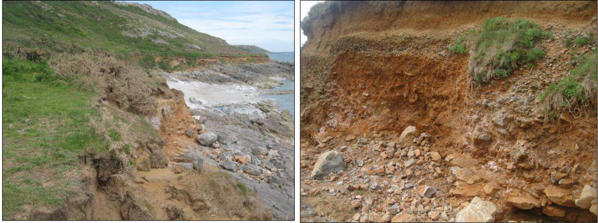
Figure 42. Small-scale erosion at Horton Cliff (Mike Howe, June 2014).
